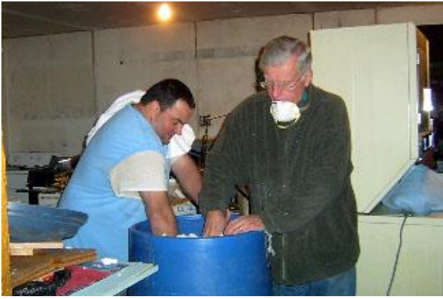
Mike Humphrey & Ed Vang load fiberglass insulation into the hopper so it could be blown above the ceiling.
