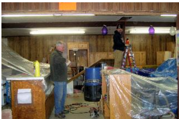
After creating a hole in the ceiling to get to a leak, our volunteers insulated the ceiling on the west side of the store. Here Ed Vang & C J Leetch get ready to blow.
