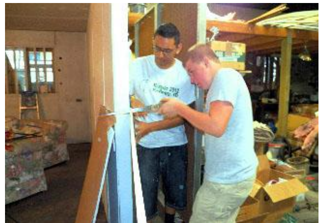
Verne was delighted to find someone with the Pilgrim Lutheran youth group who had installed wall board. Here they are covering insulation in a back room at the ReUse Store where a furnace will be installed.
