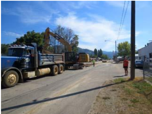
The ReUse Store was closed for more than a week while Main Street was completely torn up and repaved. Nice to have the new smooth road.
