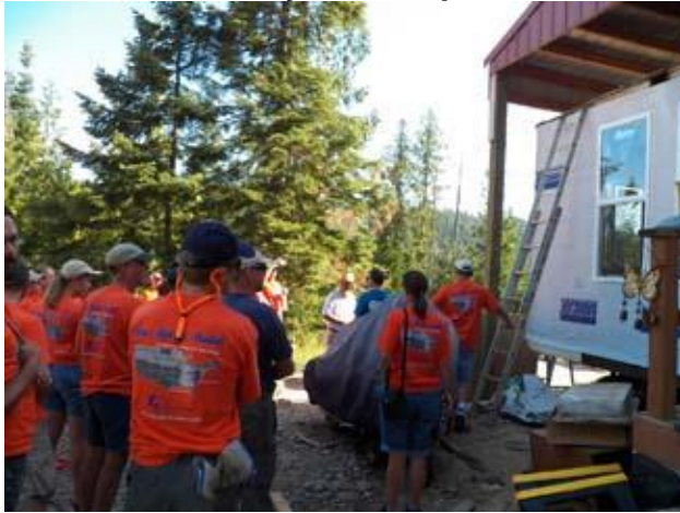
Verne greets the Fuller Center Bike Adventurers at the Mace home where they installed siding on the house.
