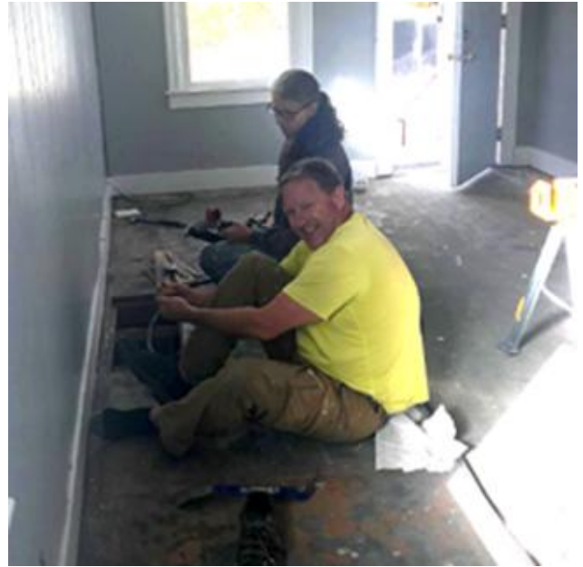
Shawn and Teresa Truelove install trim. Shawn is our Construction Supervisor. Photo by Tami Atkins
