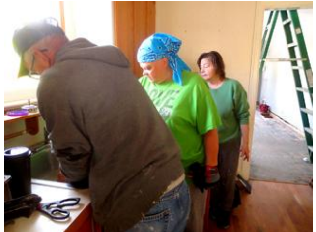
Using his janitorial skills, John Boy Delaney clears out the junk plugging the kitchen sink. Tami Atkins and Kay Baker are ready to help when possible. Photo by Judy
