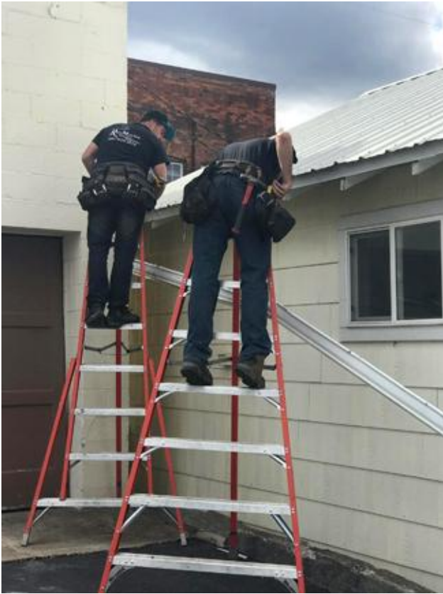
Rain Masters install seamless guttering along Kay Baker's future home Photo by Tami Atkins
