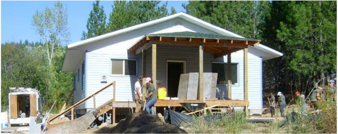
U of I students work measuring wall board at left, digging an electrical trench in front, sloping the soil away from the house at right and installing wall board inside the Lake's family home.
