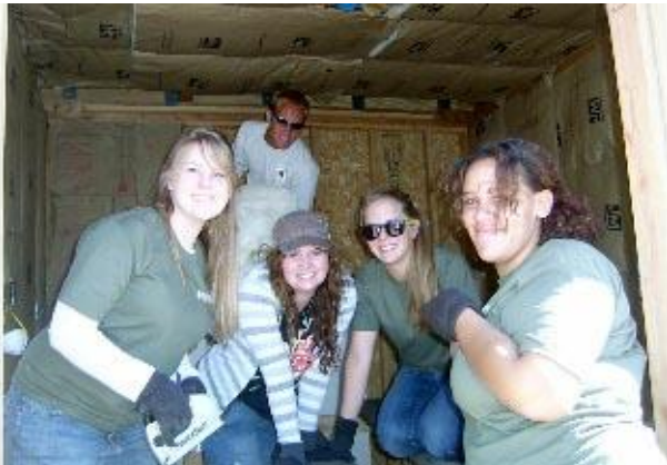
University of Idaho freshmen volunteer to help finish the “Little Shop” building that we are raffling. The drawing will be held after $4000 worth of tickets is sold at $10 each or 6 for $50 (about 400 tickets).
