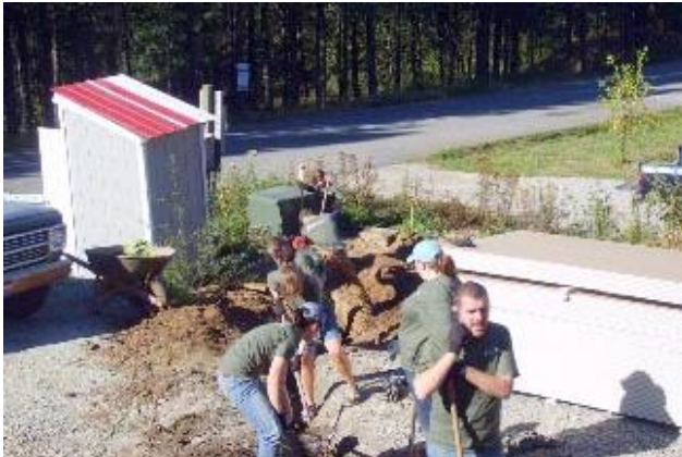
University of Idaho students dig a trench so AVISTA could lay an electrical line to the Lake home.
