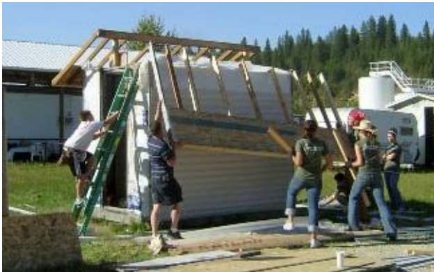
U of I volunteers and Adam Hutchings help roof and side a storage shed with Kevin Hutchings's supervision.
