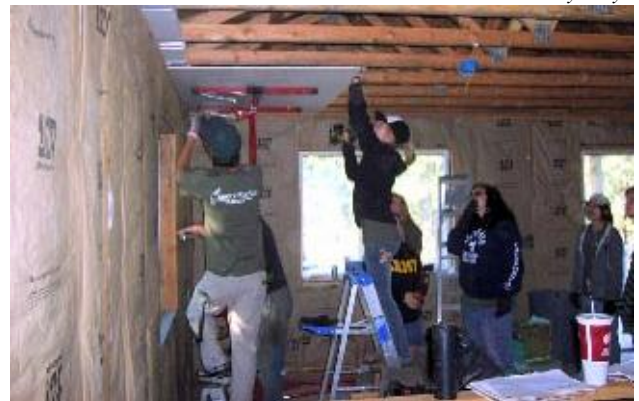
Under Jim Taylor's supervision, U of I students install sheetrock on the ceiling and walls at the Lake site.
