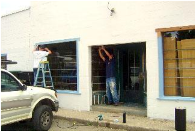
Rick Gilbert, of R&R Construction, and his helper Michael Bodine donate their labor finishing painting the front of the ReUse Store (formerly Larry's Saw Shop) in Smelterville.
