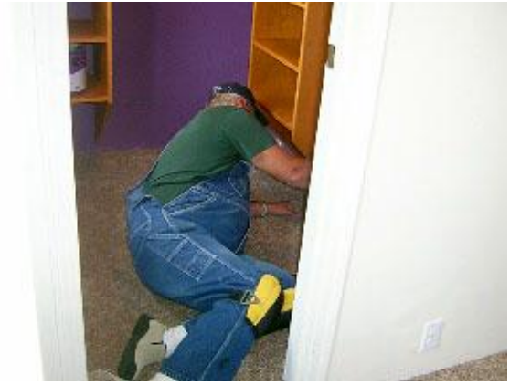
Swede Little finishes laying carpet in the Kriedeman home. Dedication of this home (our 18 th ) will be Oct 19 at 5:30 PM, 204 Hill Street, Smelterville.
