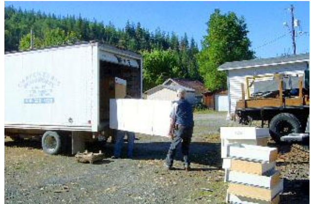
Dennis Carpenter, of Carpenter’s Woodworks, delivers cabinets taken from Silverwood Good Samaritan Center’s kitchen. Top cabinets are priced at $10 per linear foot & the base cabinets are $20 per linear foot.
