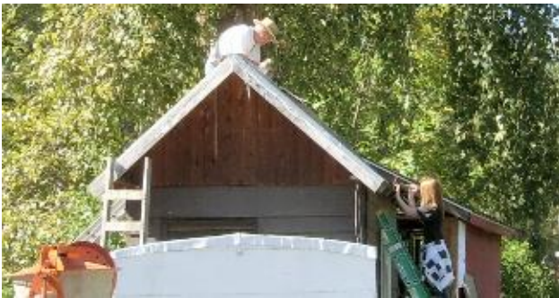
Penny Welsh stands on a ladder at right to help Verne repair the roof of the shed built by Jim Shadle. We use the shed to store windows.
