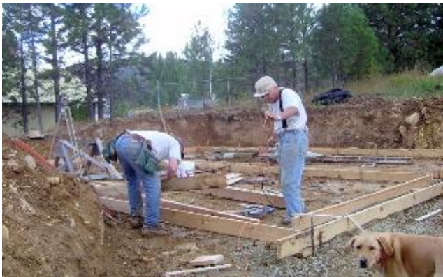
Rick Gilbert and Verne Blalack build footing forms at Sunny Slopes for the Kriedeman home. Sadie supervises.
