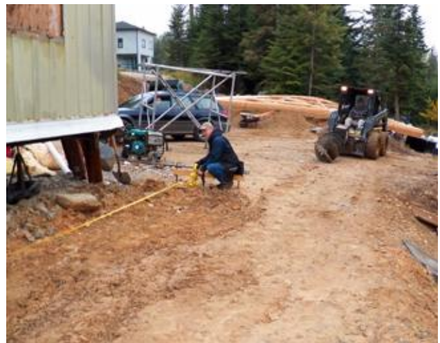
Marty Fisher holds the line at the northwest corner while the auger operator waits for the holes to be marked.
