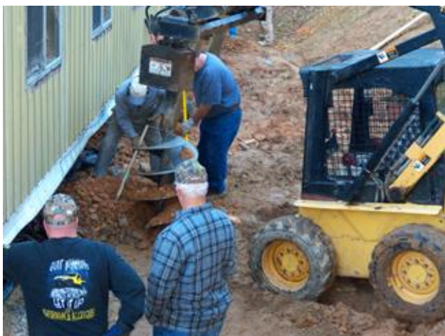
A hole drilling auger makes quick work for setting the support posts. Scott Stovern, Wally Sherwood, Dave Weingart, Don Ferguson
