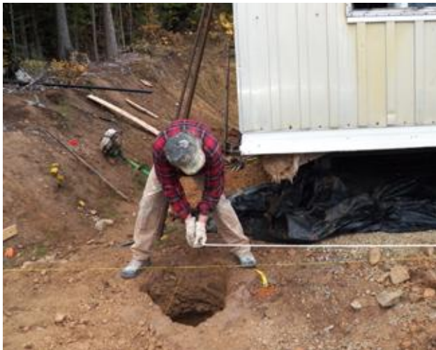
Glenn White measures the first hole on the northeast corner of the building.
