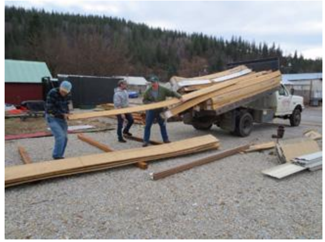
Verne Blalack and Scott Stevenson work with Ed Stice to unload a large donation of siding from Lifetime Roofing and Siding.
