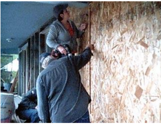
Amethyst Pelham works with Kevin Hutchings & Swede Little putting a new wall on the front of the Mullan home.
