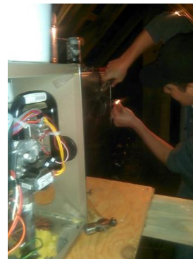
Jonathan Crawford helps his dad, Jeff, install the new furnace in the Osburn house (John Boy's future home).
