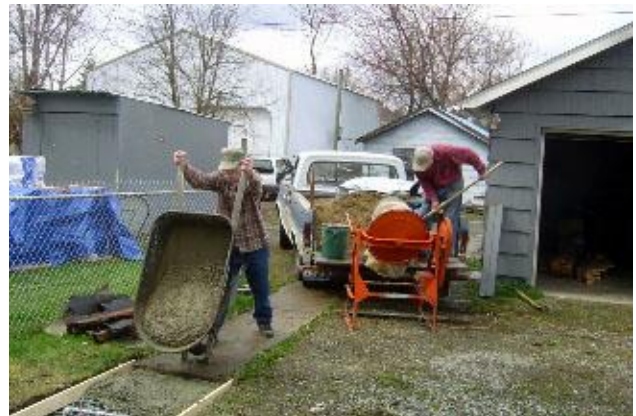
Bob Larson and Verne Blalack pour a new rear sidewalk after Don Ashcraft installed the forms at the Kriedeman home.
