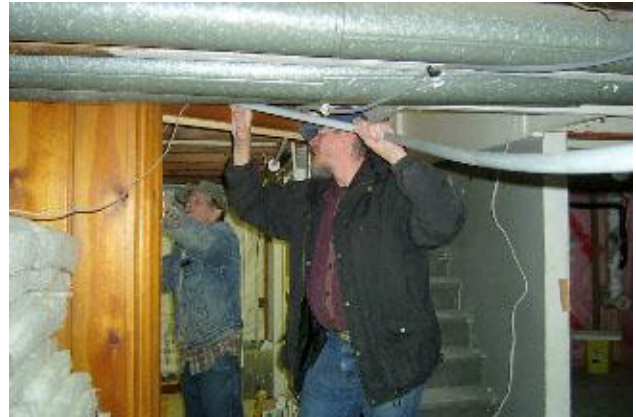
Don Ashcraft bends down to help Bob Larson thread an electric cord through conduit in the basement of the Kriedeman home. The whole house had to be rewired to fit code.
