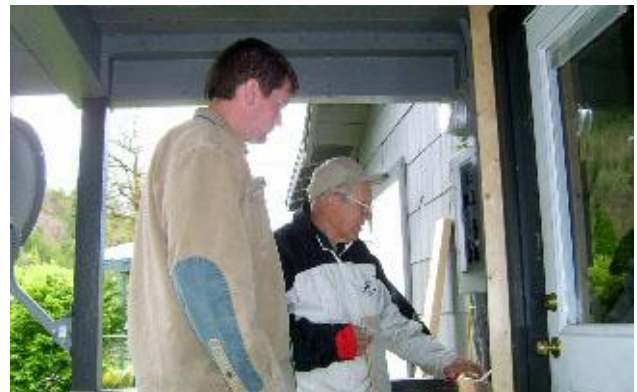
Josh Haralson of Crown Electric checks the wiring with Verne at the Kriedeman house before an official inspection is called. Photo by Judy
