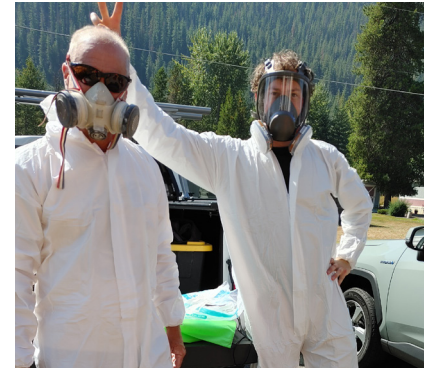
Volunteers from the Ma'Or Foundation suit up for demolition work at the trailer in Osburn
