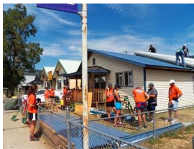
Some of the Fuller Center Bike Adventurers help a crew of Idaho Servant Adventurers from the Shoshone Mountain Retreat. They are working on the Greater Blessings roofing project at the Larson home in Kellogg. The other Bike Adventurers were installing siding at the Mace home.
