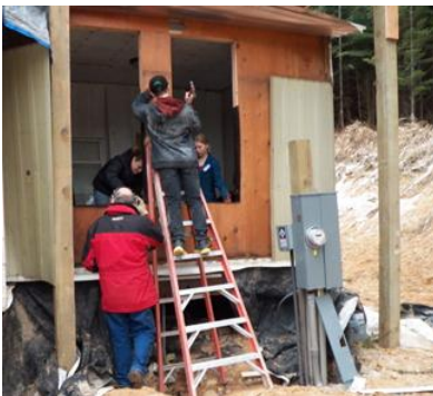
Rick Wood supervises as the Mace children, Julie, Ethan and Bethany help frame around the windows. Alex was busy inside framing doors. Rick Gilbert and Mike Humphrey were installing a matching window on the left side of the front door.
