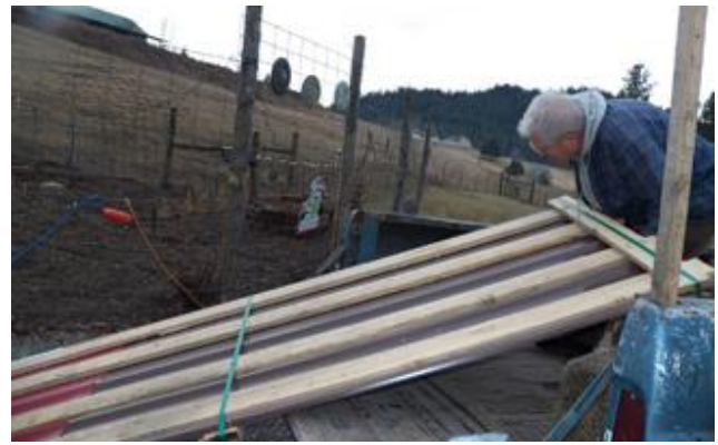
Verne drops off the metal skirting to go around Debbie Bornitz's trailer. This will be another project finished in the spring when we have volunteer helpers. Work has been completed under her home winterizing her pipes to keep them from freezing.
