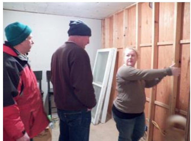
Rick Wood and Rick Gilbert watch as Christina Mace shows where the two windows need to be placed in a bedroom wall.
