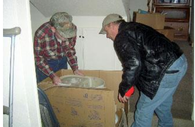
Bob Larson and Steve Critchfield installed a handicap toilet at the Coak home as a “Greater Blessings” project.
