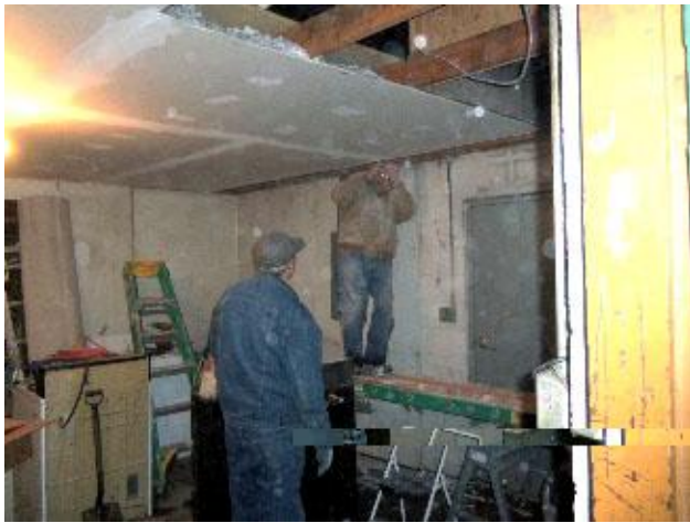
Norm Holtz and Verne work on the ceiling of one of the back rooms at the ReUse Store. Photo by C J Leetch
