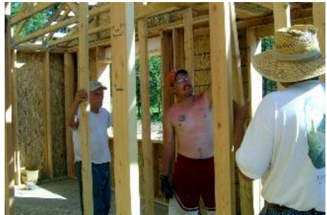
Bob Larson, Nathan Lake, and Verne Blalack discuss the interior framing at the Lake home.
