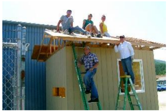
A Youth Group from Colorado staying at Shoshone Base Camp helps Bob Larson install the sheathing on the roof of our 10' x 12' "Little Shop" we will raffle. Photo by Judy
