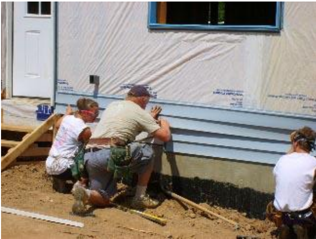
Rick Gilbert, of R & R Construction, teaches the youth from Shoshone Base Camp how to install siding on the Lake home. Photo by Mike Humphrey
