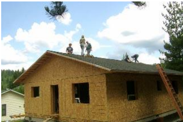
Jim Taylor, of Taylor Made Construction, supervises a Servant Youth Group from Shoshone Base Camp as they install roofing on the Lake home. Photo by Ed Vang
