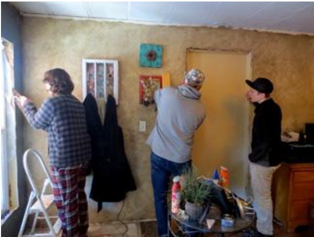
Rick Gilbert, center, shows the Mace family how to install interior window and door frames. Nathanael begins on a window at left and Ethan is watching on the right.
