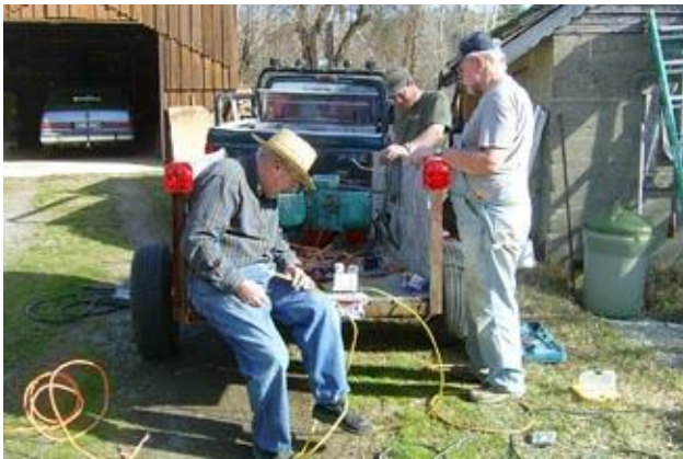
Verne, Kevin & Swede wire a generator on a utility trailer that was donated several years ago by Dana Hammond.
