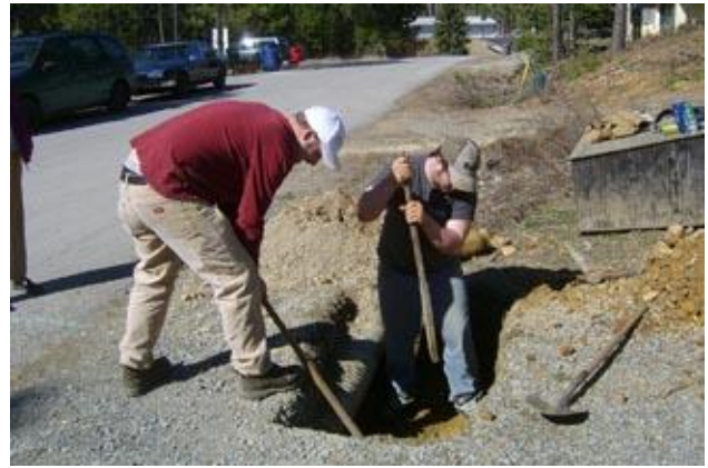
Cousins, Chris & Jake Leetch dig for the sewer pipe at the Kriedeman site.
