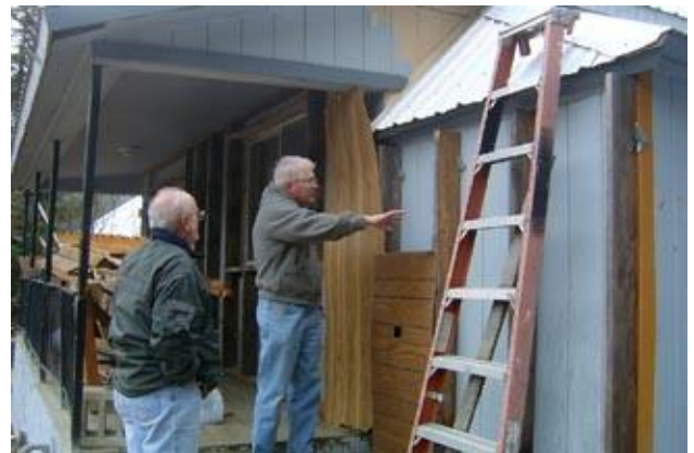
Moe Pellissier, Site Selection Committee member, listens as Verne explains how they plan to build an insulated exterior wall around the Pelham home. They will also raise and insulate the roof above the bathroom.
