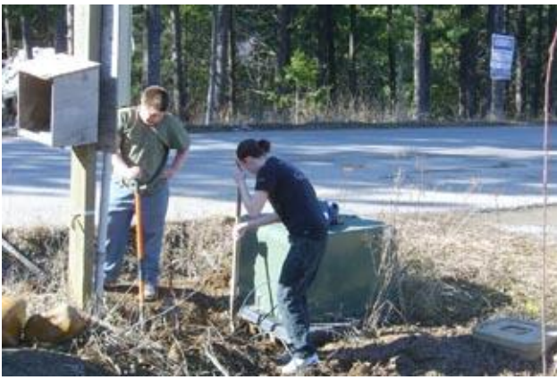
Adam Hutchings and Mara Ashcraft dig out the temporary electrical pole from the corner of the Lake property so it can be reset at the Kriedeman site a couple lots west.
